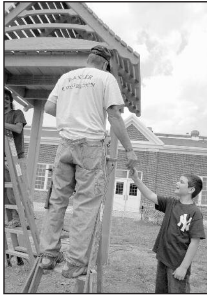
3rd grader John Otters helps a crew from Baxter Construction working on Hopewell's new bell tower.
